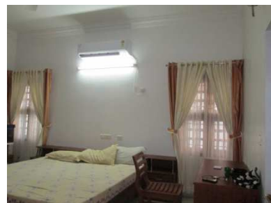
Figure 124: bed room with mechanical cooling
