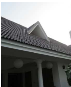
Figure 123: gable as an aesthetic element only
