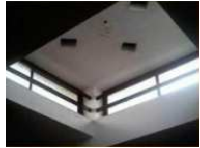
Figure 88: roof top air vents
