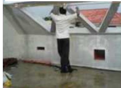
Figure 86: air vents and wind trapping system above the roof.
