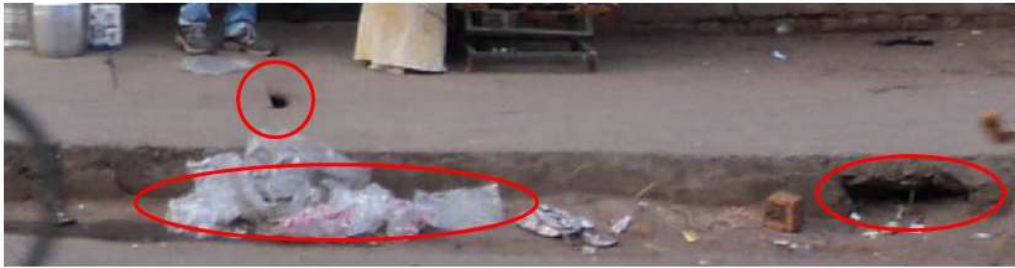
Clogging of drain and improper maintenance
