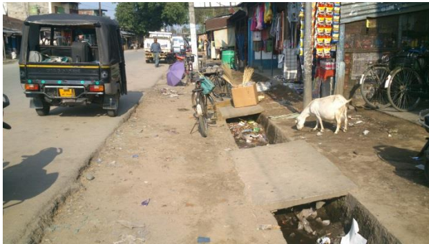
Clogged drain in the market area
