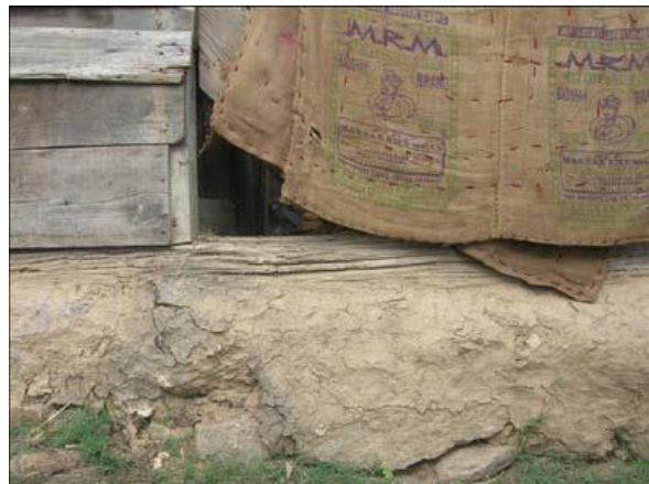
Figure 17: Stone foundation rising above ground level, in a typical thathara house - village Rohta, Distt. Chamba (H.P.)
