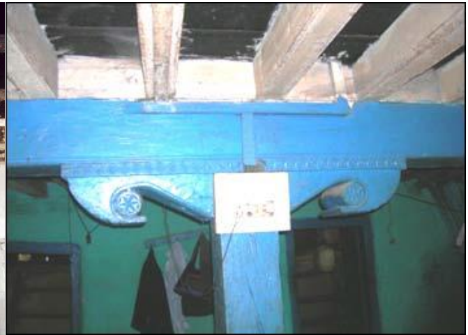
Figure 26: Main beam supported over wooden post (thamb) in the middle of the room
