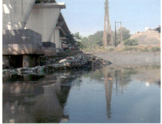
Figure 4.12: Blocked water way below 100 MLD Saket bridge
