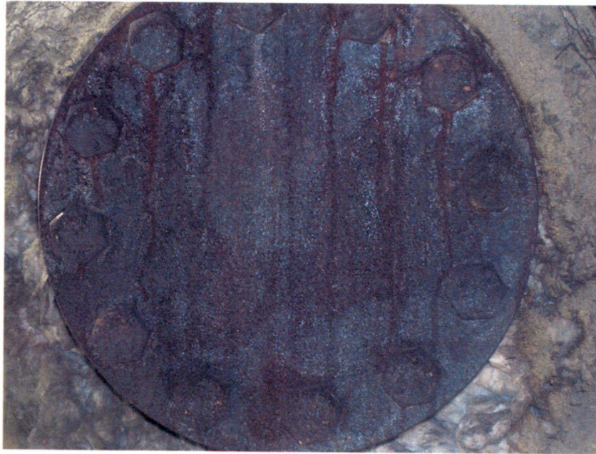
Fig. 4.12: Unlagged steam pipe flange
