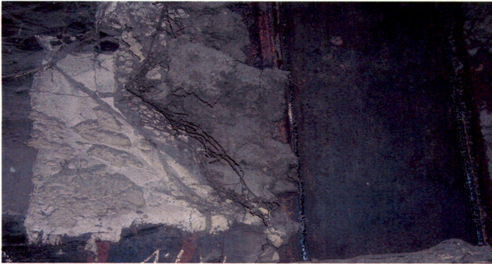
Fig. 4.14: Unlagged steam pipe
