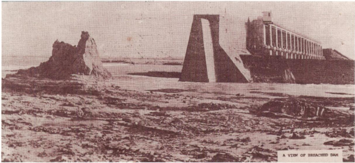
Figure 1.1: A view of breached dam
