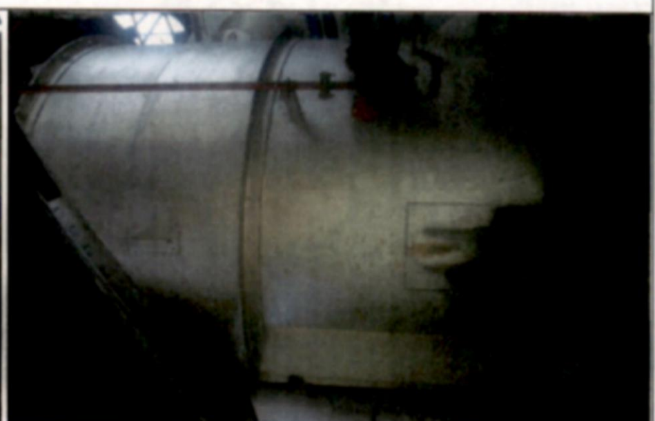
Fig. 5.12:INCINARATOR (OUTSIDE VIEW)
