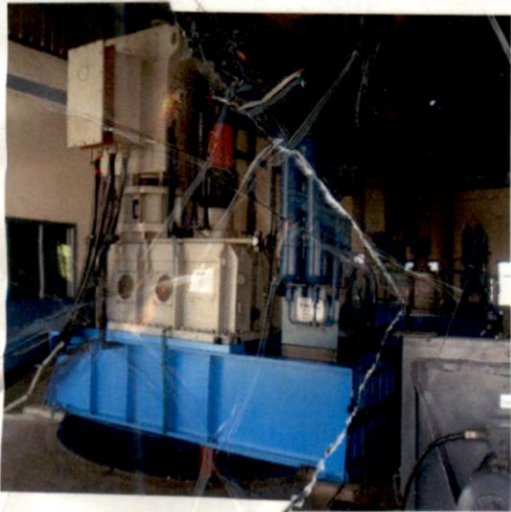
Induction generator at Dolowal SHP
