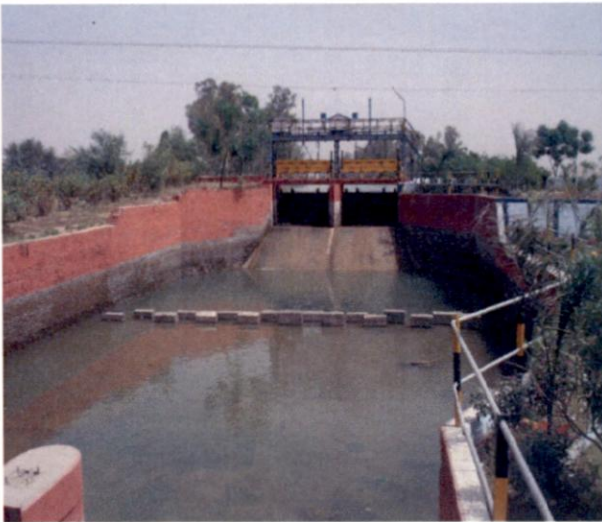
Intake at Babbanpur SHP
