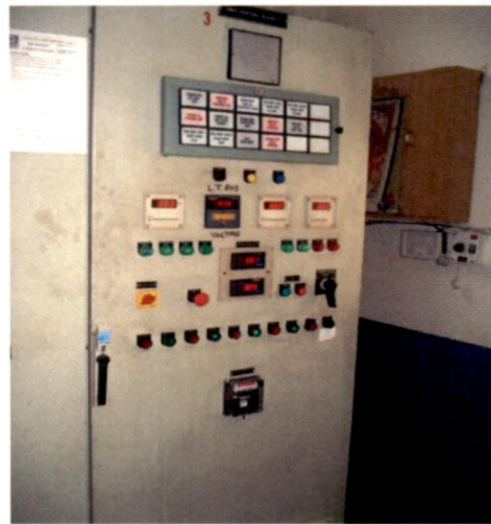
Unit Control Board at Salar SHP
