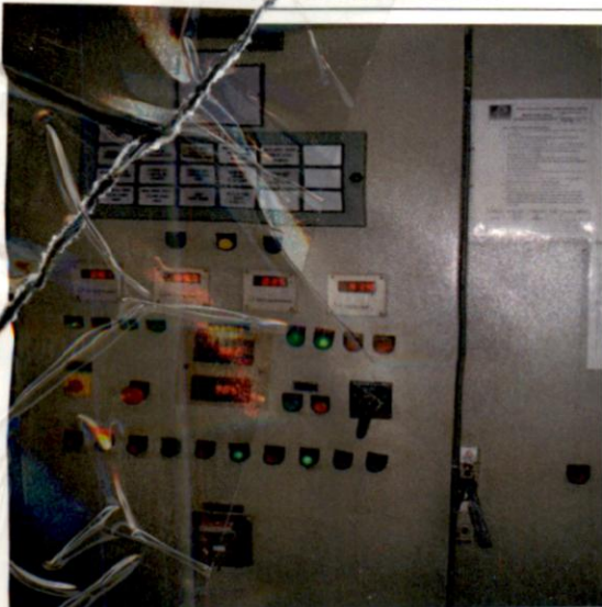
Unit Control Board at Dolowal SHP
