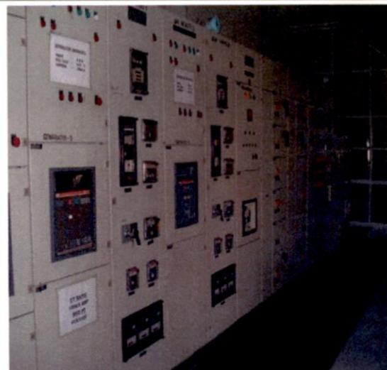
Control room at Banbhaura SHP
